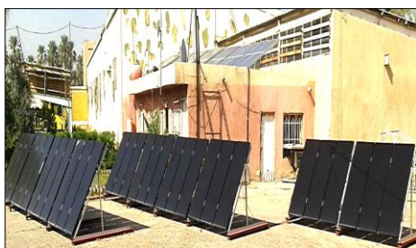
Figure 1: View of current PV solar system
